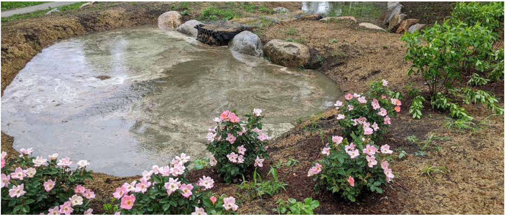
This infiltration basin, built in 2019, is designed to reduce phosphorous loads by 11.6 lbs/year rather than being discharged directly to the ponds at Roger Williams Park.
